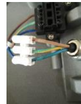
Connect power wires
